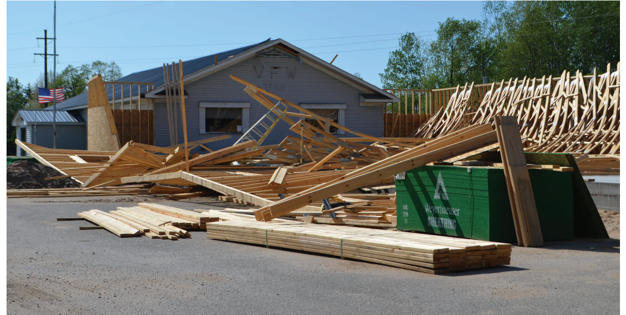
High winds were to blame for the collapse of a building under construction last week at the former VFW Hall on M-32 just south of East Jordan. The hall is being remodeled and to accommodate the new Crossroads Resale shop, which is planning to expand its business and move from its current location in East Jordan. PHOTO BY KRISTAL JOHNSON
